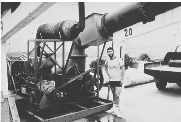
Figure 34. One of 20 large intake pumps at farm in Salinas, Ecuador.
