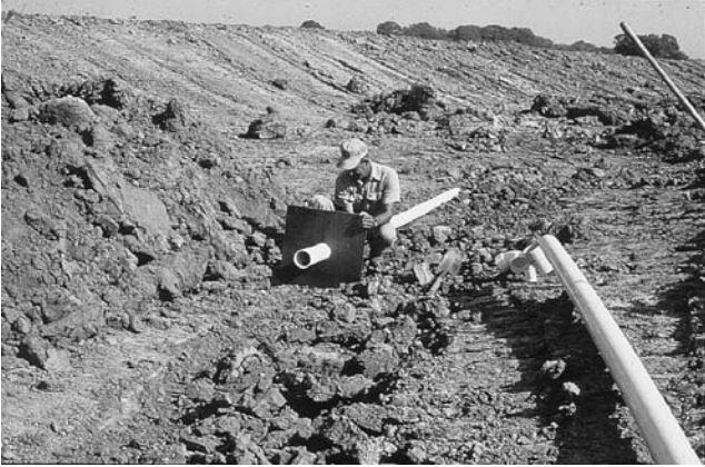
Figure 4. An antiseep collar (this one fabricated from metal) being placed around a drain line that will be installed through the levee of a pond under construction.
