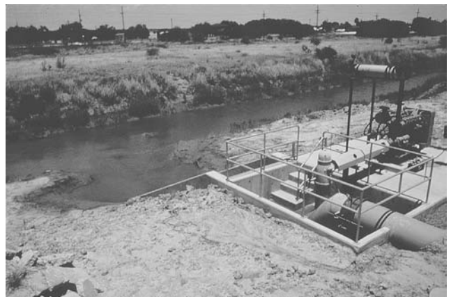
Figure 17. Recirculation water pump at Arroyo Aquaculture Association farm in Texas. (Photo by Louis Hamper.)
