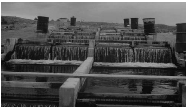
Figure 4. Raceways are often constructed side by side, with common walls. In some instances, the raceway units may be stair-stepped down a hillside, as shown at Leo Ray's fish farm (Buhl, ID), in order to provide some water aeration before serially reusing the flow in downstream raceways.
