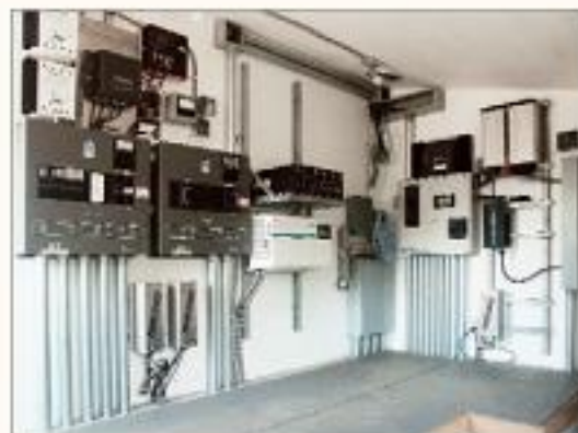
Power room, which houses our batteries, inverters, and other renewable energy equipment
